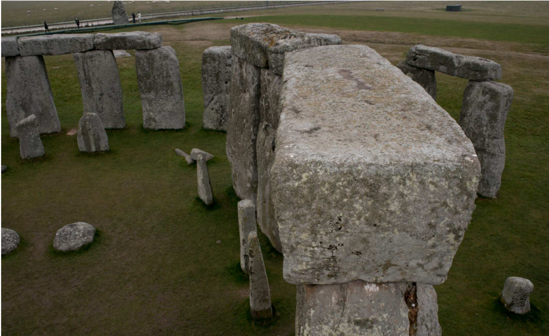
An example of the digital photography taken from the high level access boom.
